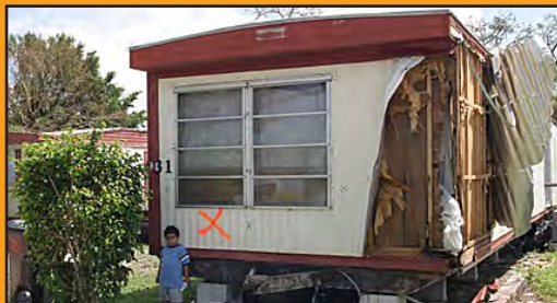
Wall coverings damaged and exposed, Mobile Home (MH)
