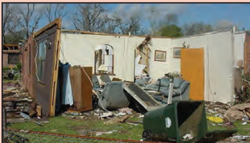
Roof gone, walls collapsed, Mobile Home (MH)
