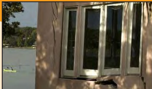
Foundation damaged, Single Family (SF)
