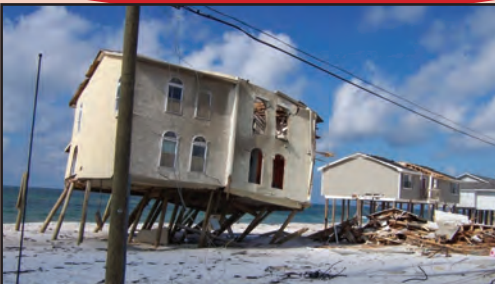
Foundation, roof, walls unsound, Multi-Family (MF)
