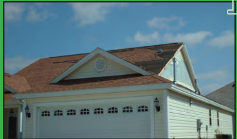
Few missing shingles, covered, no impending weather
