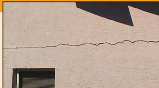
Structural cracks—roof lifted, Single Family (SF)
