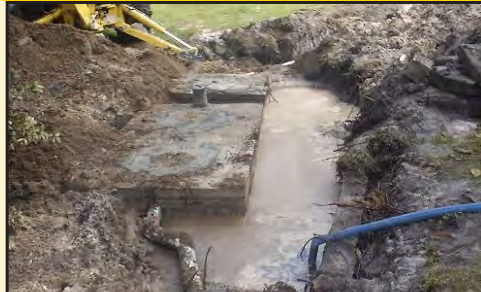
Flood septic tank damage
