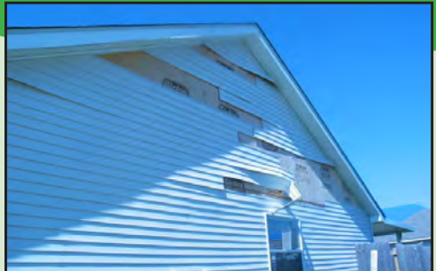
Loose and missing siding
