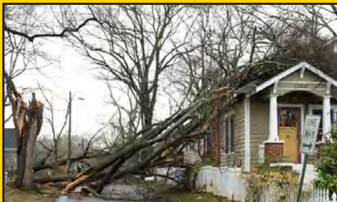
Tree on structure but no breach, Single Family (SF)
