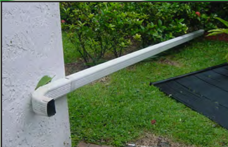
Gutter damage and debris
