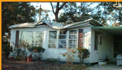
Roof partially collapsed, Mobile Home (MH)
