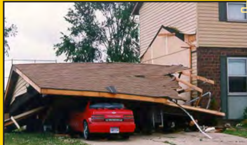
Damage to wall small breach, Multi-Family (MF)
