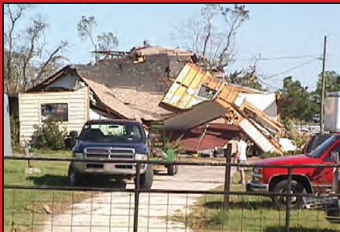
Roof & walls collapsed, Single Family (SF)
